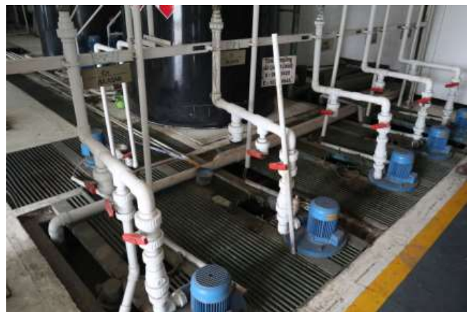
Fig. 9. Electroplating WWTP unit in weapons manufacturing and assembling division
